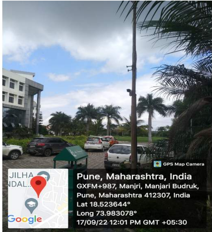
CCTV camera at College Entrance
