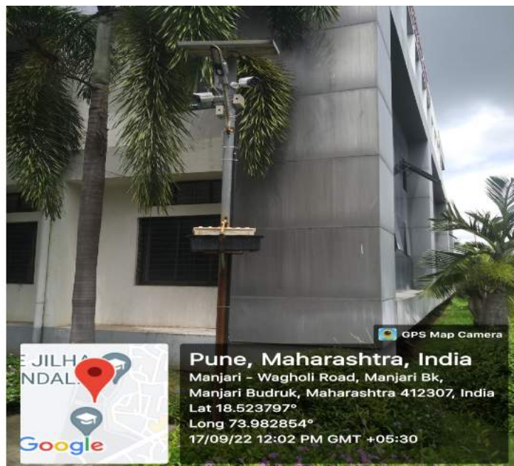
CCTV camera at A Building
